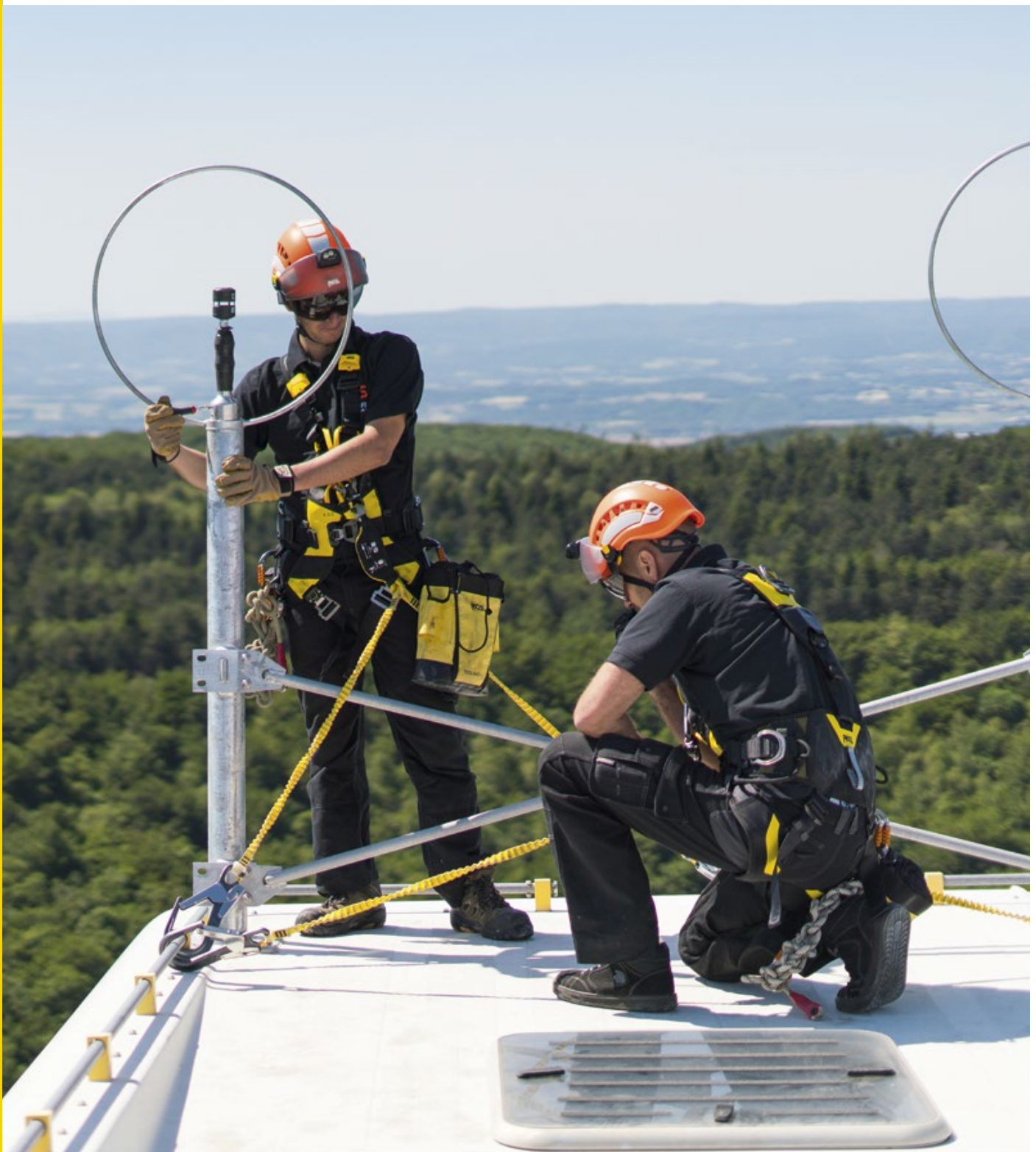
Maintenance operations of wind turbines, France © 2019 - Petzl Distribution - Vuedici.org - RES - Parc éoliens de Marsanne
