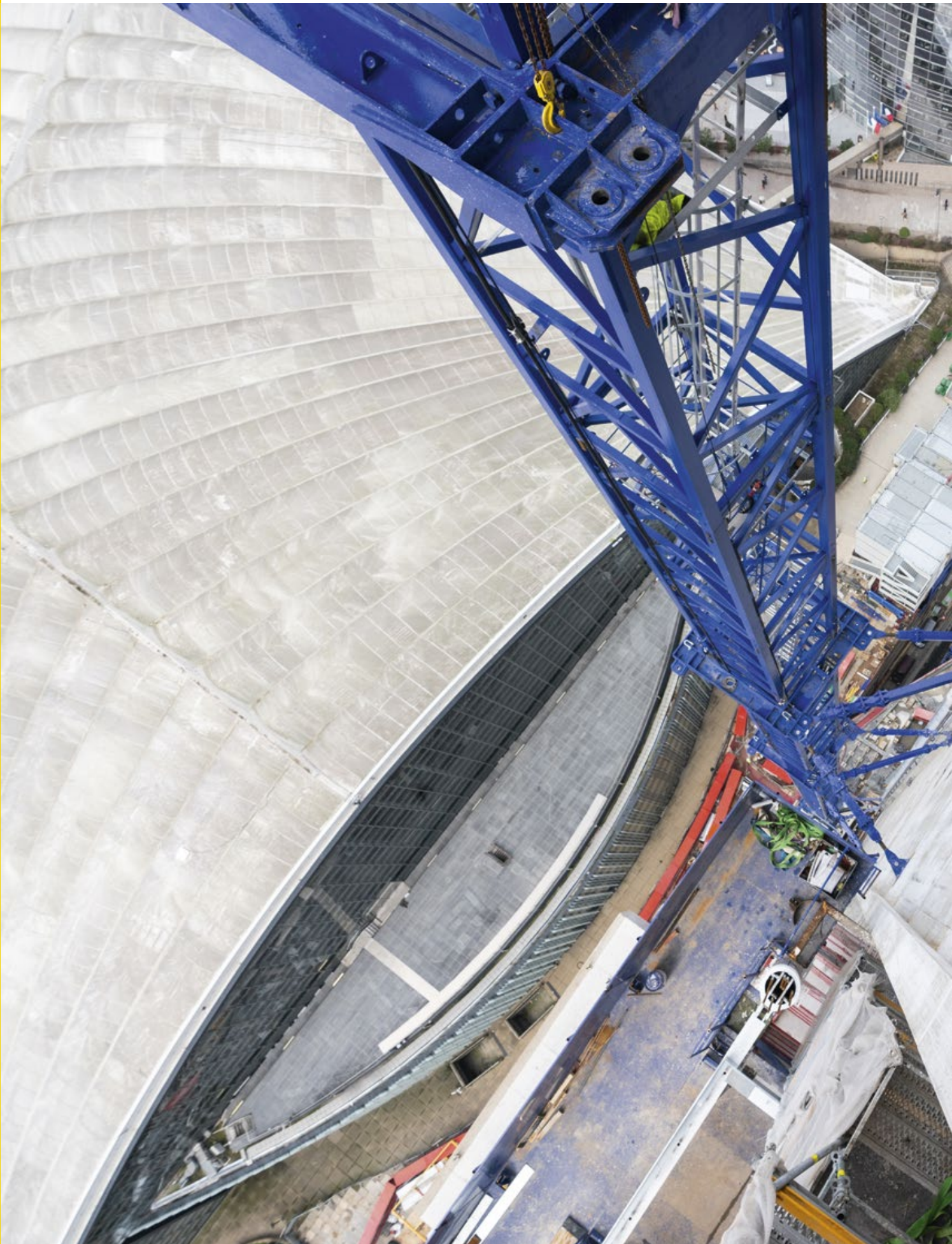
Repositioning the braces of a tower crane, France © 2019 - Petzl Distribution - Vuedici.org - Integral - Bateg - Tour Trinity - Cro&Co Architecture
