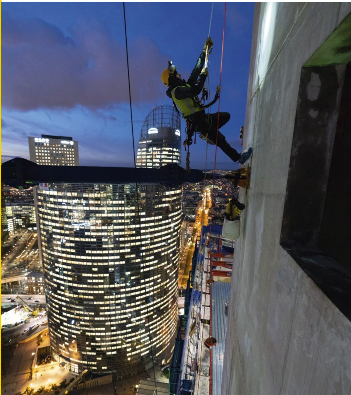
Repositioning the braces of a tower crane, France © 2019 - Petzl Distribution - Vuedici.org - Integral - Bateg - Tour Trinity - Cro&Co Architecture
